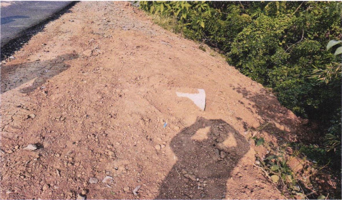
3. DFCCIL's Contractor Discharging water to private land
